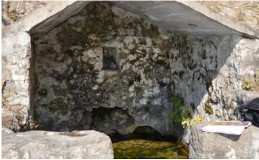
Two natural water resources (Bavaris) selected for repair and revival and hygiene, Simour, HP
