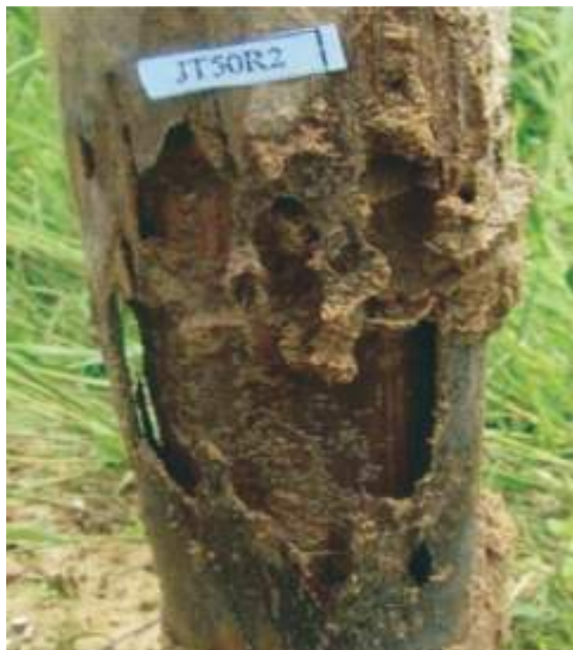
Damage to Bamboo due to Undetermined Termite
