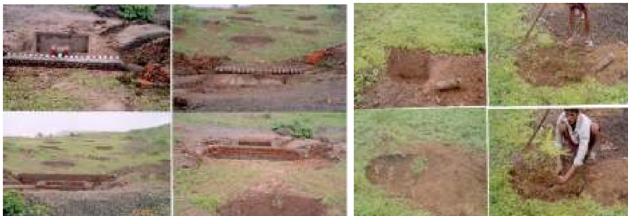
Rainwater harvesting devices (top), run-off measuring devices (lower four left) and plantation activity at the site (lower four right)
